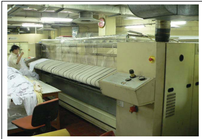
Gambar.6.9. Flat work Ironer/Mangler
